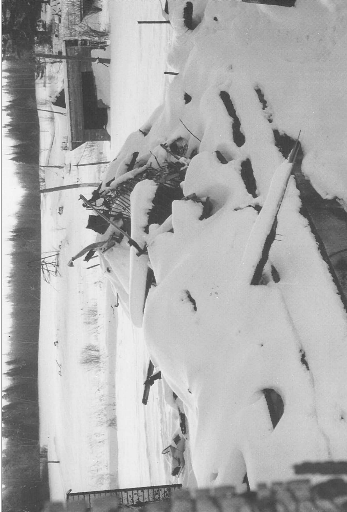
12. View of basement area showing extensive debris and remoteness of the property.
