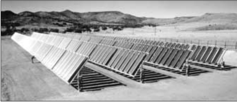
ENTECH's 100-kW high-efficiency concentrator PV system, modified under NREL's PV Manufacturing R&D project, operates reliably for the Central and South West Services Solar Park in Fort Davis, Texas.
