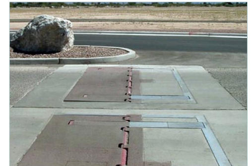
Figure 3-2. Pop-up barrier in down position at Davis-Monthan Air Force Base
