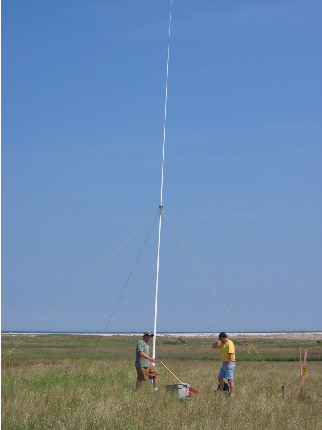
Figure 4. Long range HF Radar Transmission Antenna located on Cedar Island, Virginia during field testing activities held in June 2005.
