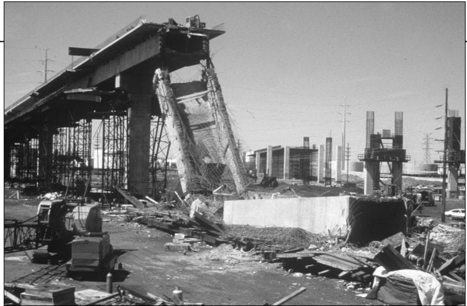
Collapse of a concrete highway ramp under construction.
