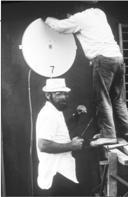
Richard D. Marshall, research structural engineer, with Philippine Weather Bureau technician installing a pressure transducer to one of the wind test houses at the Quezon City, Philippines field test site.
