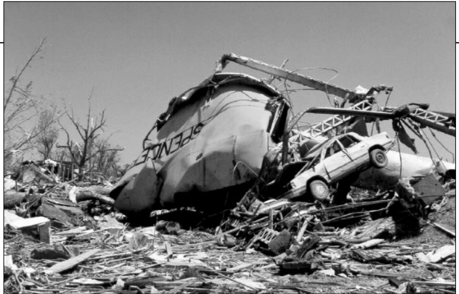
Collapsed steel water tower in Spencer, South Dakota due to the May 30, 1998 Spencer tornado.
