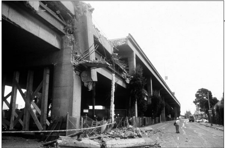
A failure of supporting columns resulted in the collapse of the bi-level I-880 Viaduct during the 1989 Loma Prieta Earthquake in the San Francisco area.
