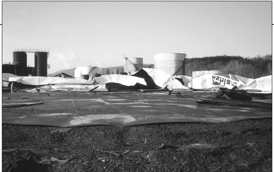
Brittle fracture propagation occurring in tank caused it to rupture and spill its full contents into the neighboring Monongahela River.
