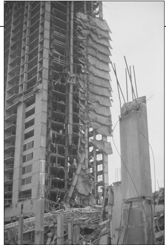
The progressive collapse of this apartment building under construction was triggered by the failure of an upper story floor as a result of premature removal of formwork.
