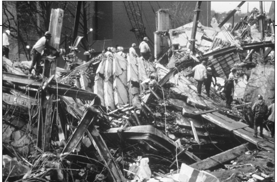
Appearance of the L'Ambiance Plaza apartment building that collapsed during construction.
