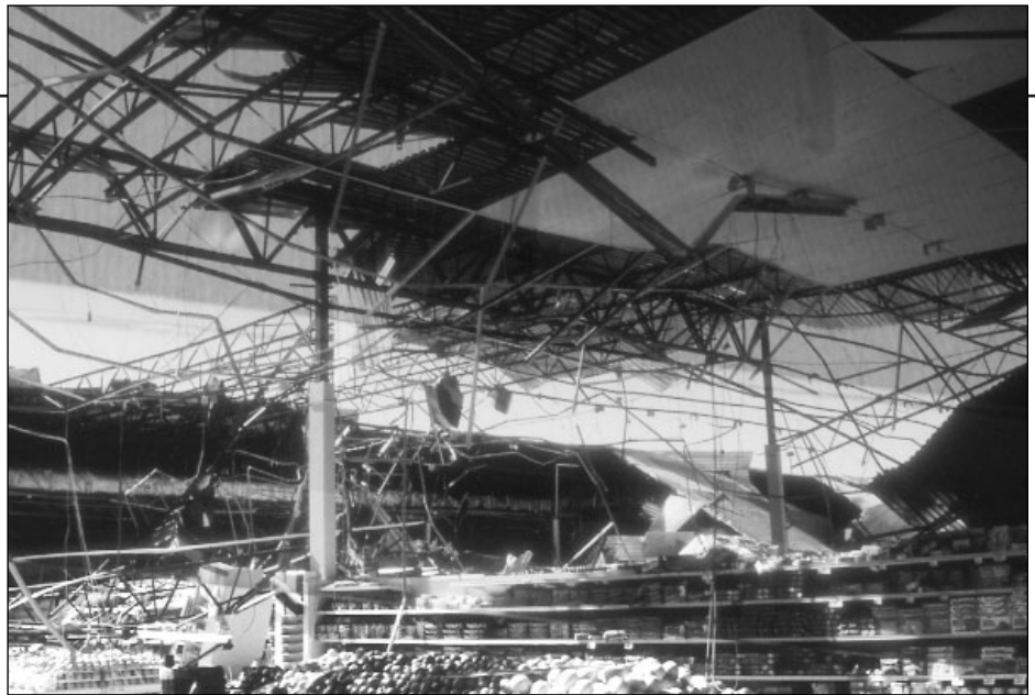
Structural damages to low-rise commercial and residential constructions caused by the 1997 Jarrel, Texas tornado included the partial collapse of the roof of a supermarket. The roof was supported by open-web steel trusses.
