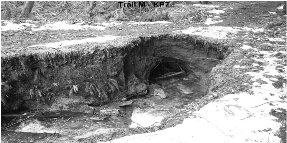
Figure 1: Failed stream crossing on Trail M
