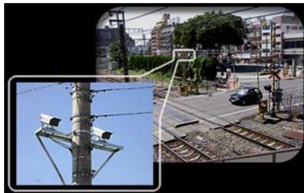
Figure 15. JR-East Stereo Camera System at Crossing [16]
