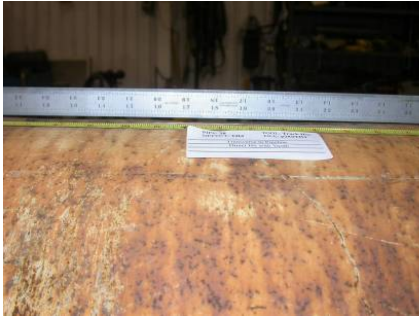
Figure 3-15. Defects D7, D8, D9 (p28dTH4)
