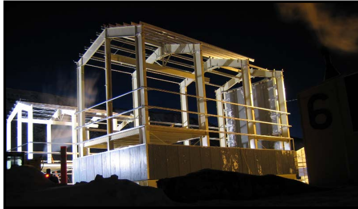
Above, the framework for the two payload buildings rises in the night. The buildings will provide facilities for the annual long-duration balloon projects launched from the ice near Williams Field.
