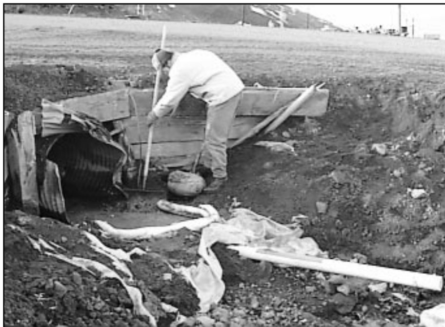
Replacing absorbent pillows that capture spilled fuel permeating from the perma-frost soil is a daily chore for McMurdo workers this season. "Its hard to say if its getting better," said Greg Lehman as he made the daily clean-up. "But it is pretty nasty stuff to get on your clothes."
