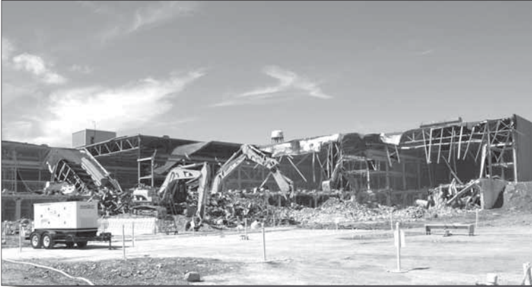
K-29 was demolished in mid-2006 as part of the Accelerated Closure Project.
