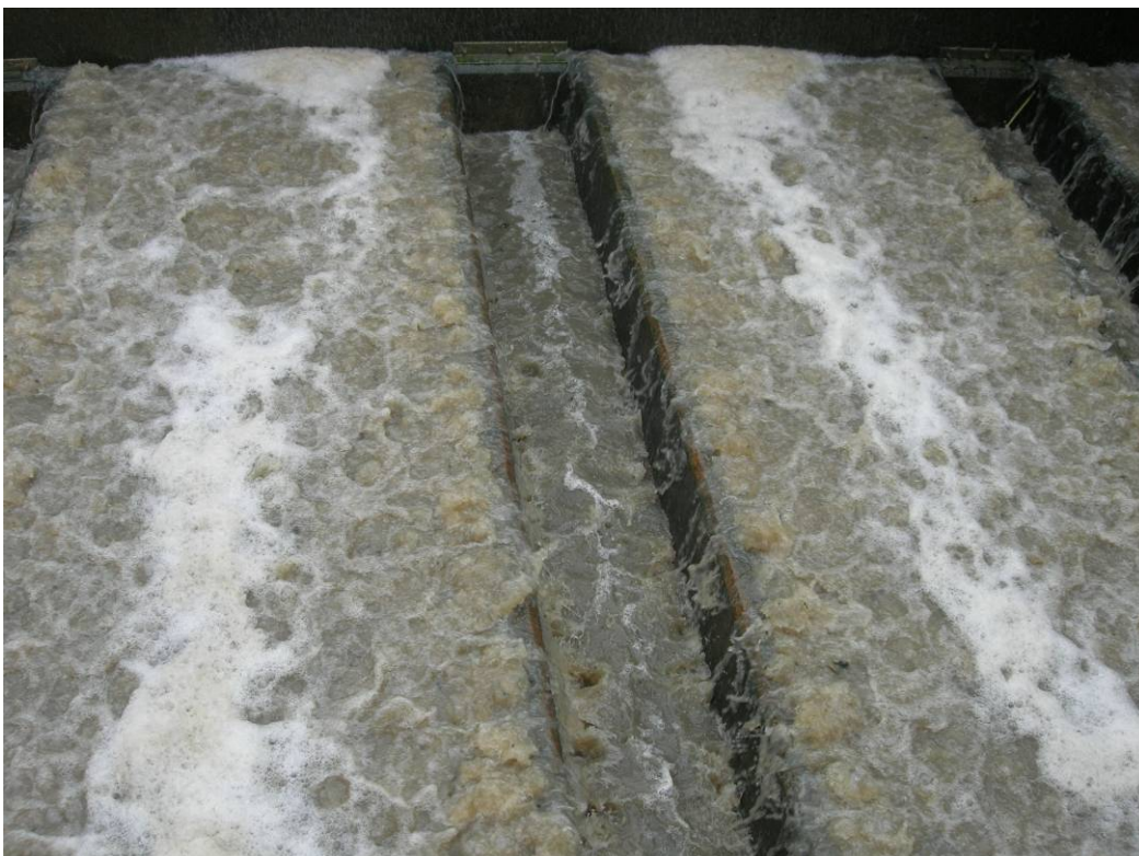
Bed filter undergoing backwash at Alexandria AWWTP
