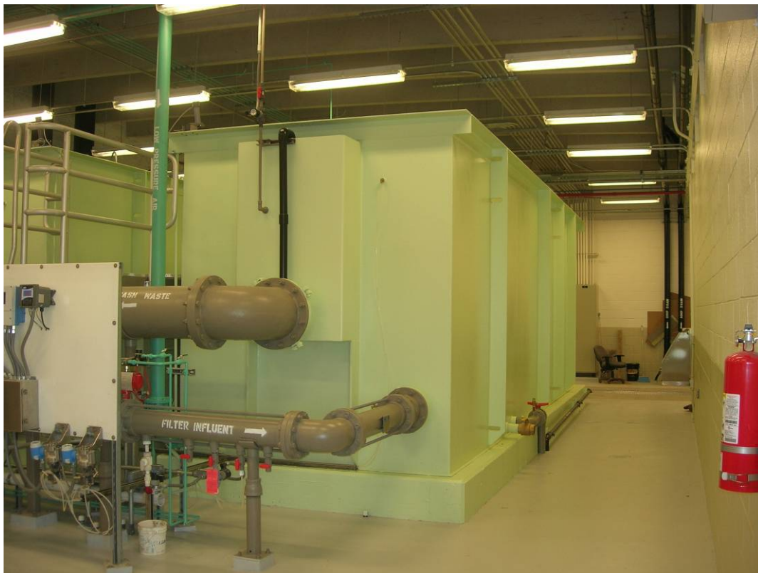
Modular Memcor Filter (US Filter Company) at Pinery WWRP. Each of these modules has a treatment capacity of approximately 0.5 mgd.
