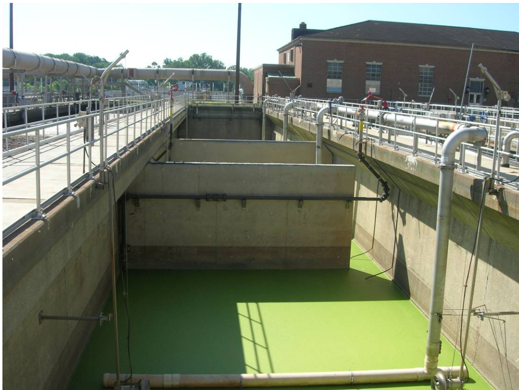
Baffles installed in wastewater contact basin (empty) to achieve anoxic and aerobic conditions for enhanced biological nutrient removal at Noman Cole PCP.
