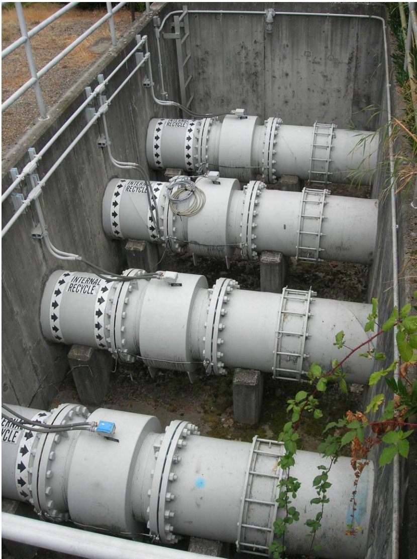
24 inch internal recycle piping at LOTT's Budd Inlet WWTP
