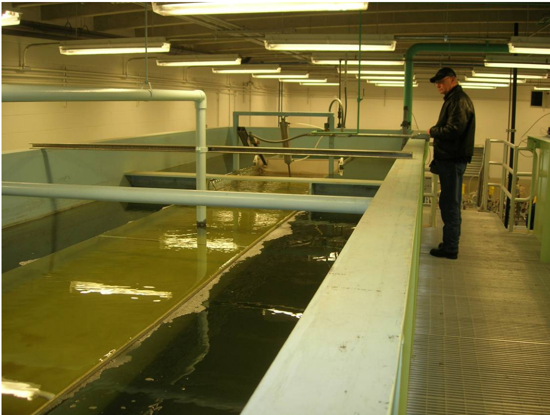
Memcor filter module at Pinery WWRP undergoing backwash
