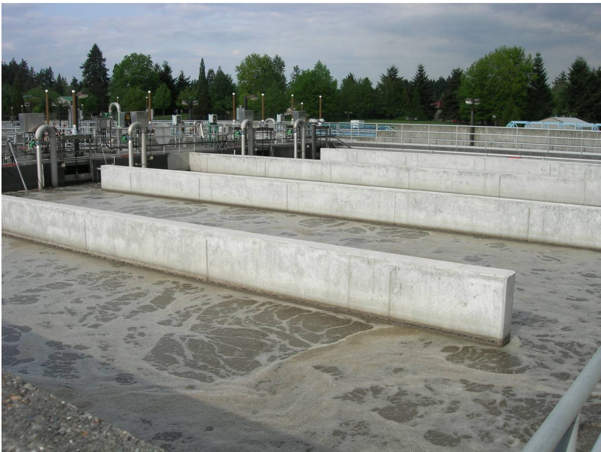
Aeration basin at Clean Water Services, Durham AWWTP. The basins at the Rock Creek WWTP may be modified in the future to also provide enhanced biological phosphorus removal.
