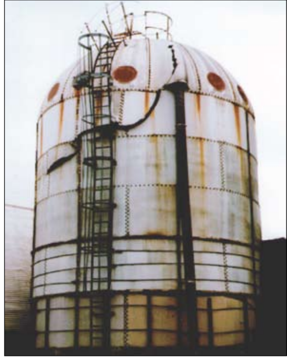
Damage to silo from explosion crack in vapor space
