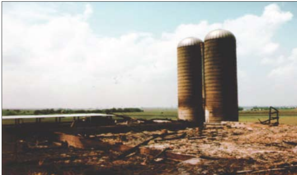
Fire originated in the silo on the right, then extended to feed room dairy barn, cattle shed, and feed
