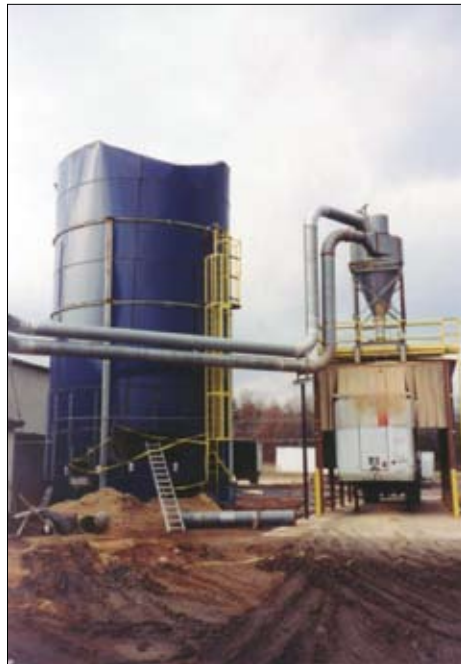
Damage to silo hatch at base; one firefighter blown onto the roof of shed at right.
