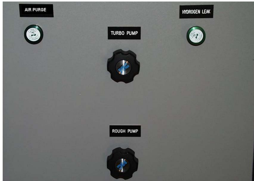
Figure 2.6. Location of Vacuum Control Valve Handles on Outside of Main Cabinet (One Set on Each Side for Each Test Chamber).
