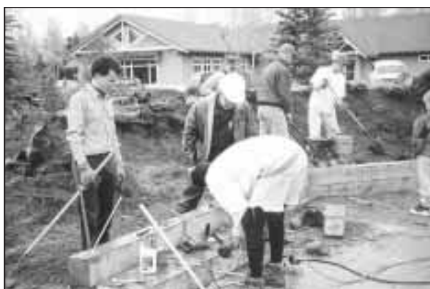
Learning about leadership and volunteering, Boy Scouts under the supervision of an Eagle Scout candidate construct an amphitheater in front of BLM's Campbell Creek Science Center in Anchorage, Alaska.
