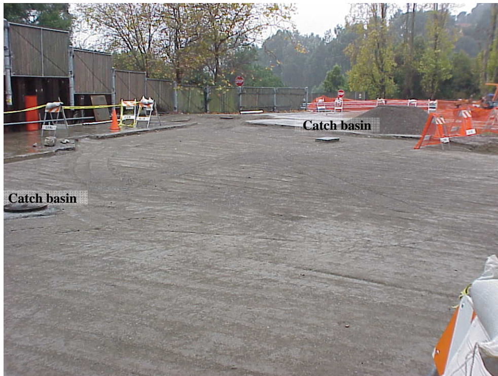
Backfilled excavation looking northwest showing the two new storm drain catch basins
