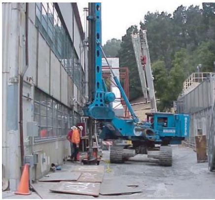
Building 64 Northeast Groundwater Collection Trench
