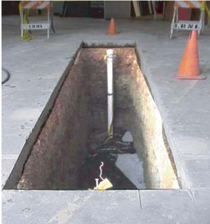
Building 64 Injection Trench
