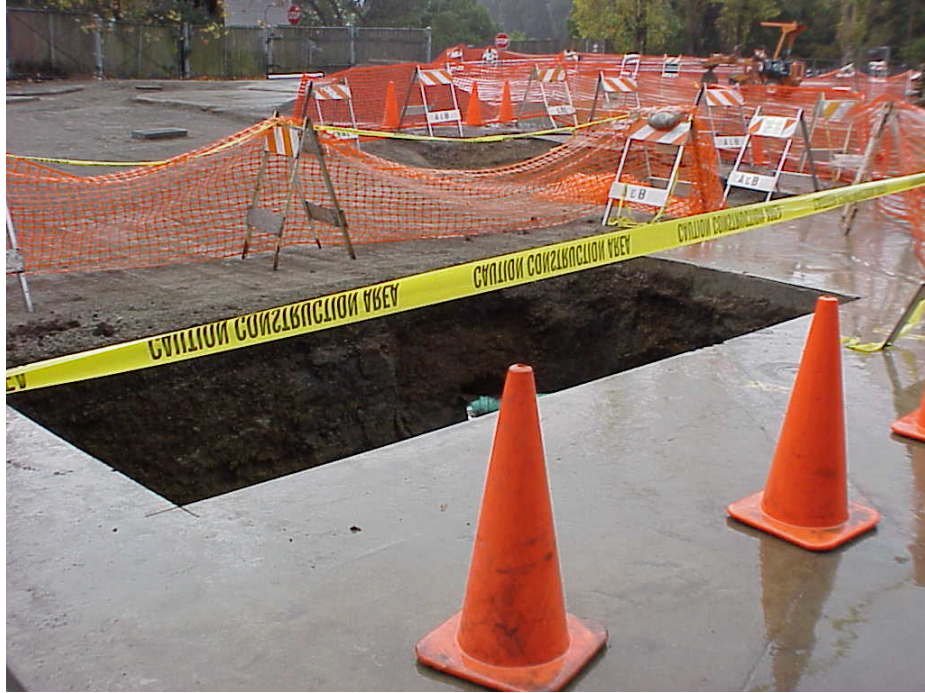
Additional excavation on east wall to remove contaminated soil detected in confirmatory soil sampling.
