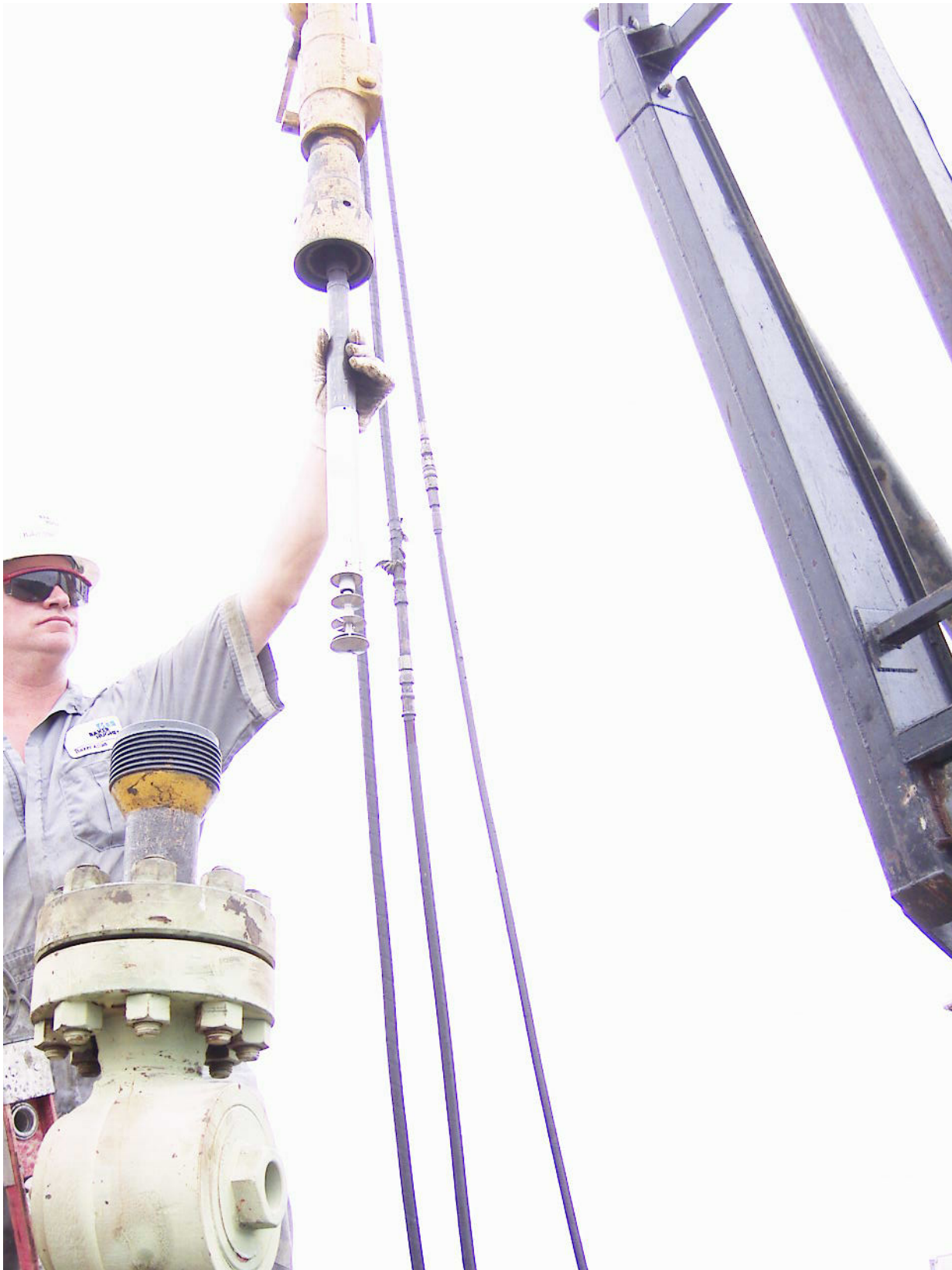
Figure 11: Insertion of acoustic tool into well
