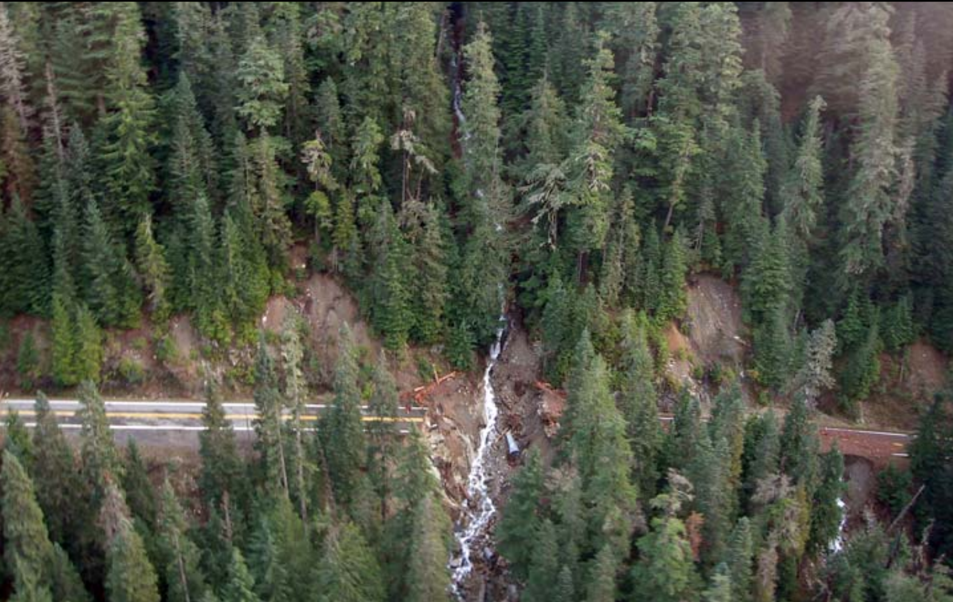
Washout at milepost 11.5 on Highway 123
