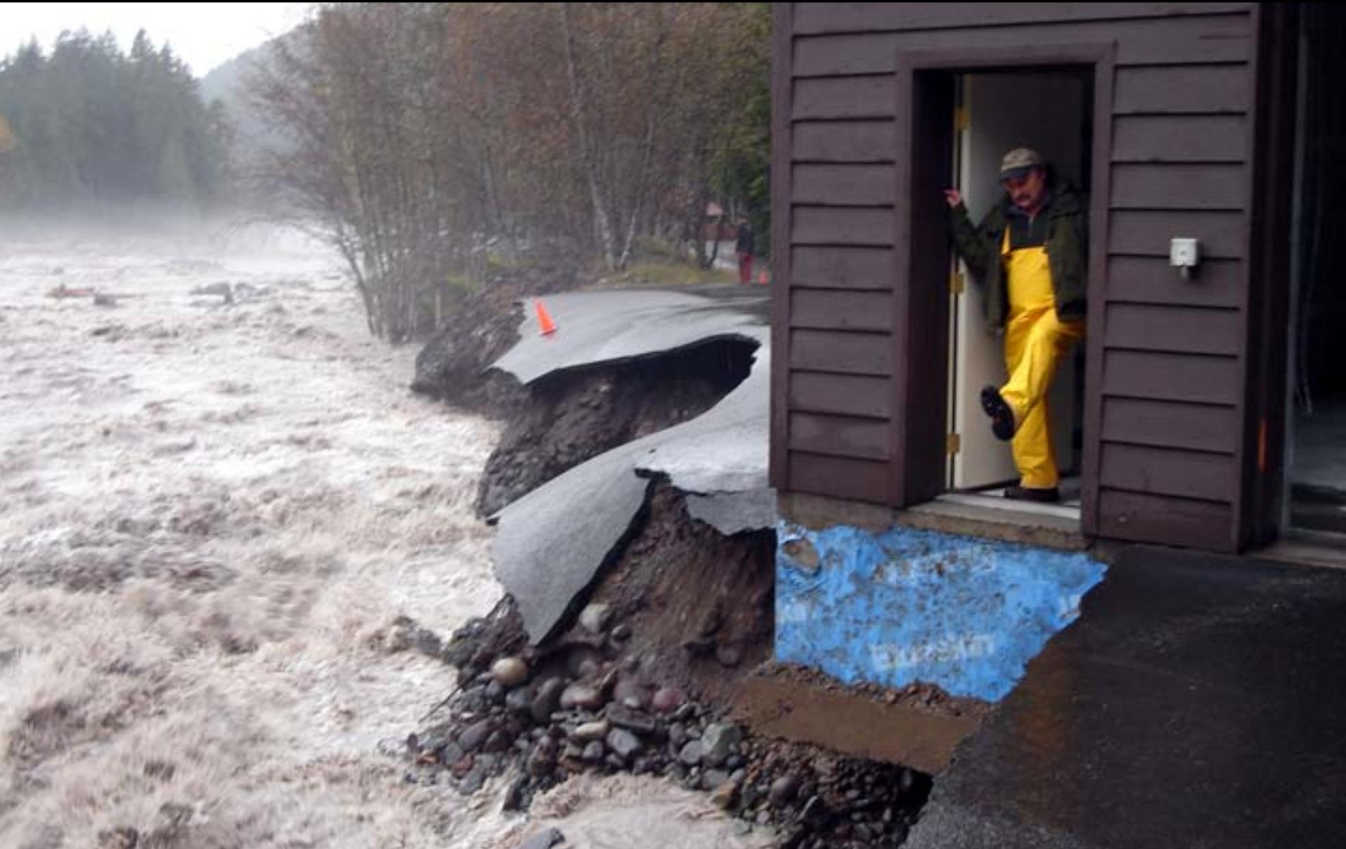
The Emergency Operations Center at Longmire, after the flood
