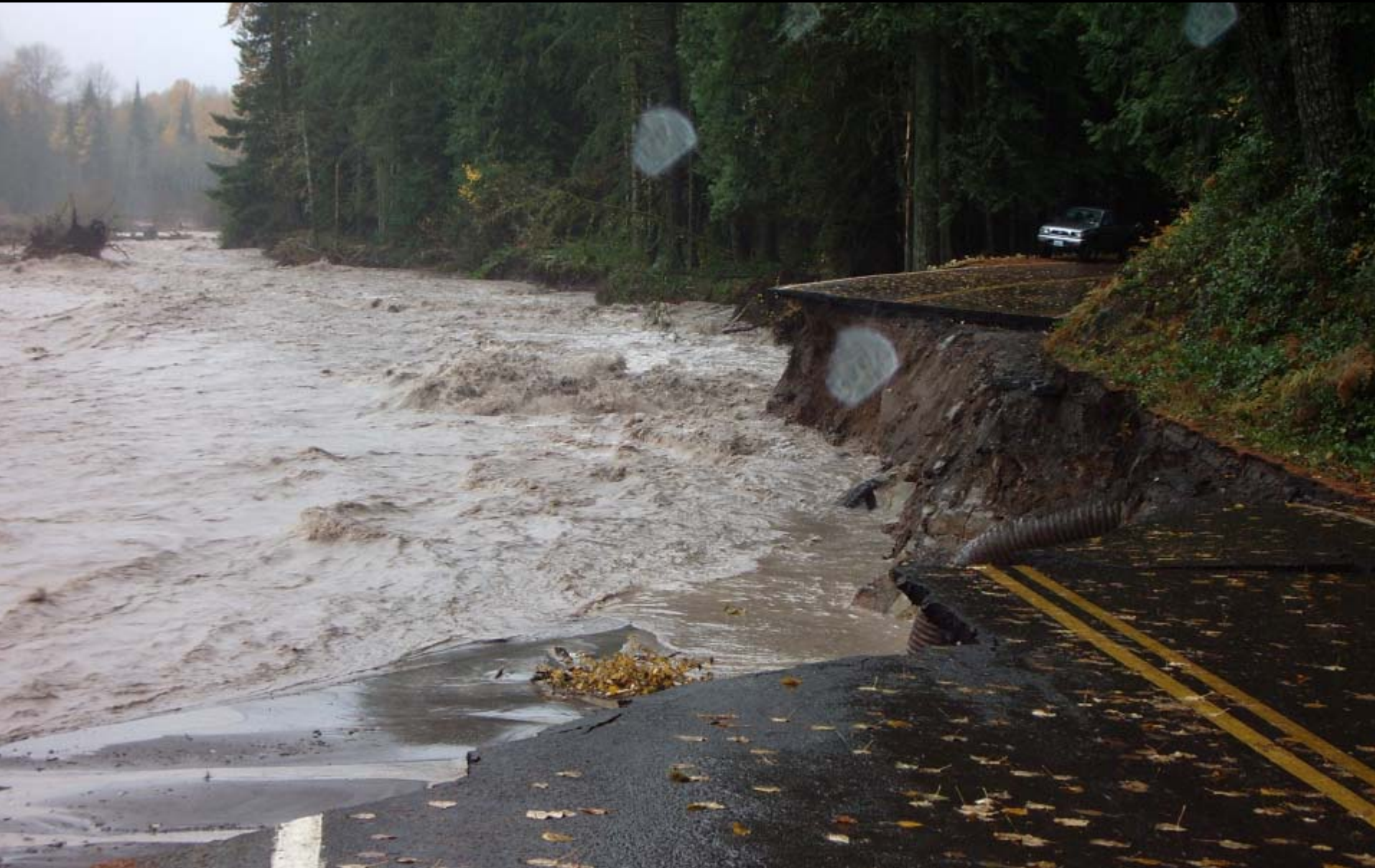
The major washout on the Nisqually Road
