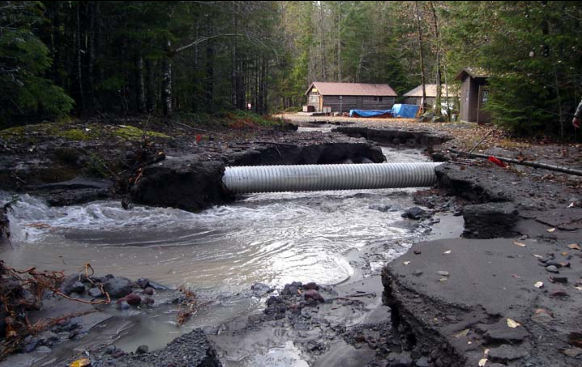
Washout at the Kautz Helibase
