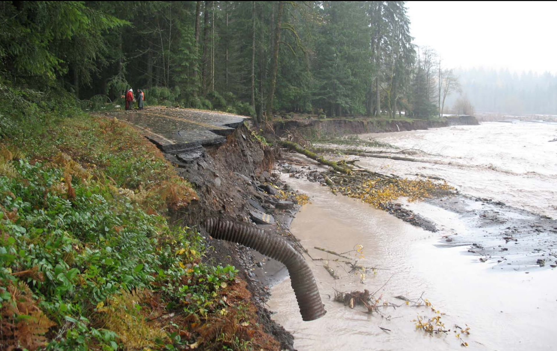
The Nisqually Road and site of the former Sunshine Point Campground
