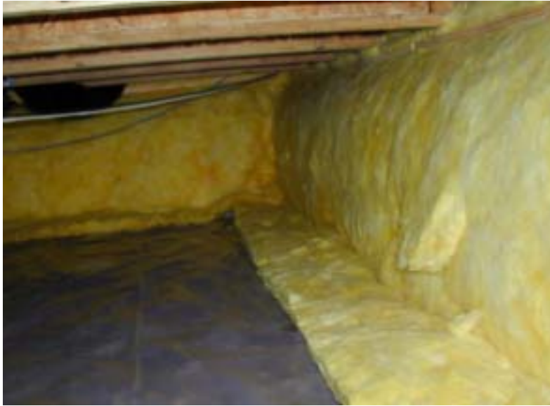
Figure 4. Unvented and conditioned crawlspaces with insulated walls are recommended. Because foundation walls of a crawlspace are usually at least partially above grade, insulating the exterior side of the walls requires detailing to ensure that the insulation is not exposed to the elements. Consequently, builders often choose to insulate on the interior side of the wall. The insulation on the inside must meet flame-spread requirements and should not have an impermeable face, so that moisture is not trapped within the wall assembly.
