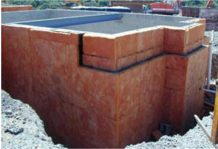
Figure 1. The semi-rigid fiberglass board insulation, 2-3/8 in. thick, provides R-10 thermal performance and water drainage at the exterior of the foundation wall. It was applied over a dampproof coating to the height of the sill plate. The exterior edge of the brick or wall sheathing above the board was designed and installed so that the edge would lay flush with the foundation wall, thereby protecting the top edge of the insulation board.
