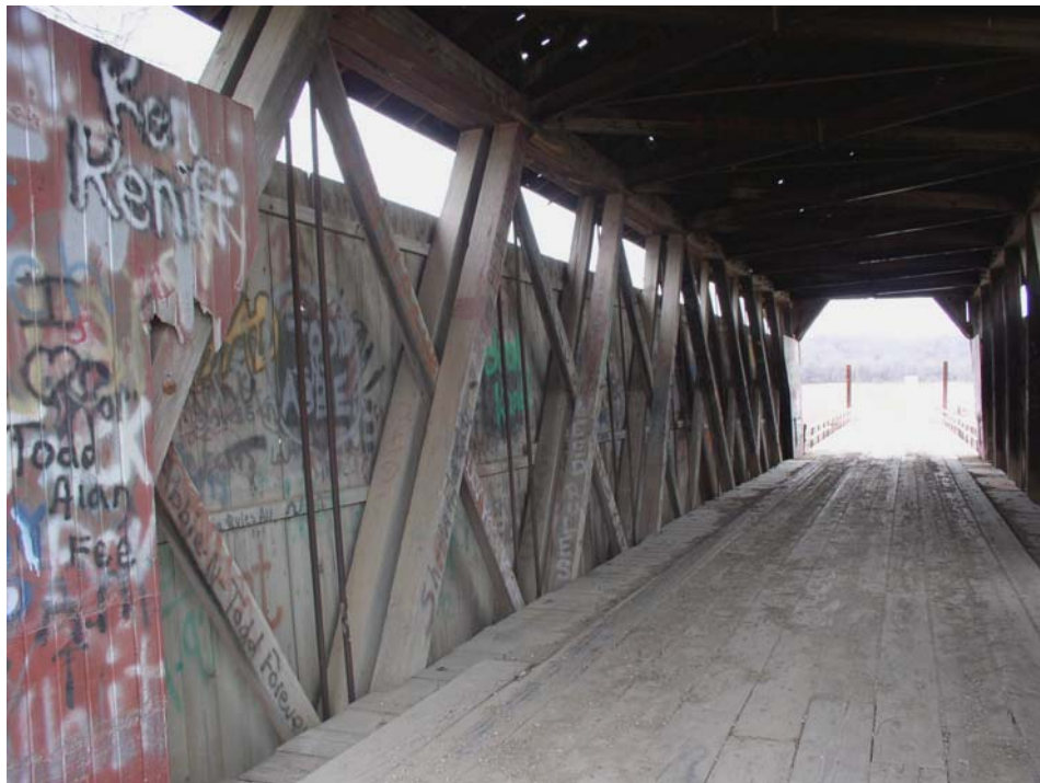
Figure 10 Pre-rehabilitation interior view of “lattice” panels or Howe truss panels, looking north from south end of the bridge. (Nash photo)
