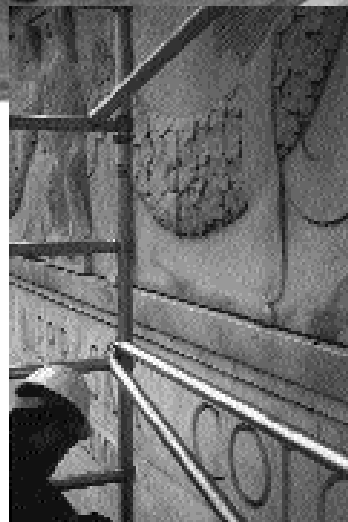
View of the attic ornamentation at the Lincoln Memorial showing deterioration.
