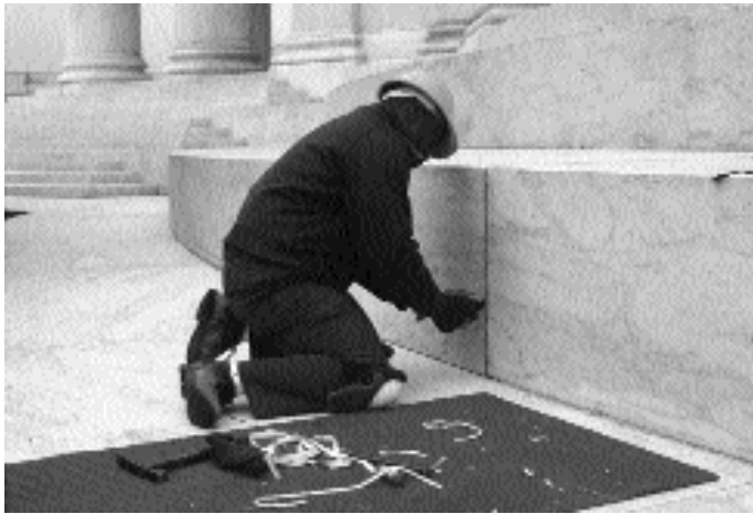
A maintenance worker repairs a stylobate joint at the Jefferson Memorial. Photo by the author.
