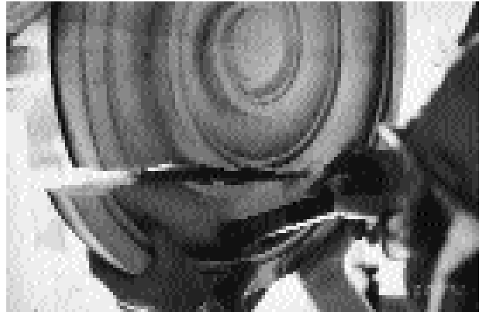
A worker removes a broken volute from a column capital at the Jefferson Memorial.
