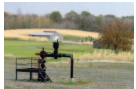
The high-deliverability Stagecoach facility is the easternmost underground natural gas storage facility in the United States. This facility was recently sold by Central New York Oil and Gas Company to Inergy L.P. The facility has a maximum withdrawal capacity of 500 MMcf/day to meet the peak gas needs of the eastern United States.
