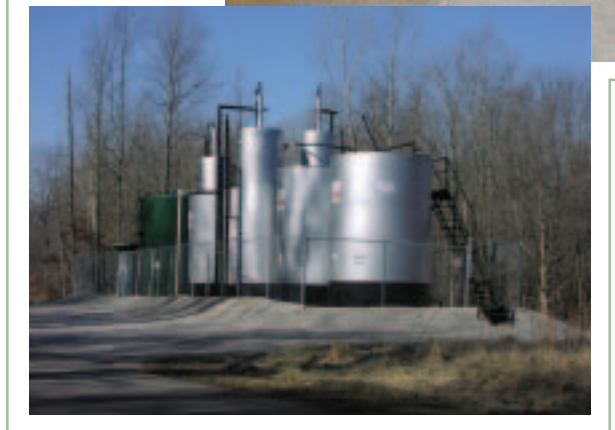
After drilling, the site is reclaimed, and the well head and fluid separation and/or compression equipment may be all that remain in the rural landscape.
