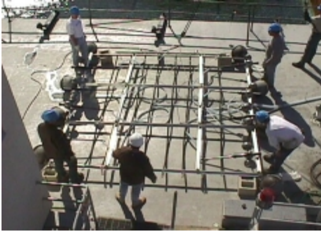
PROPANE BUBBLER SYSTEM
