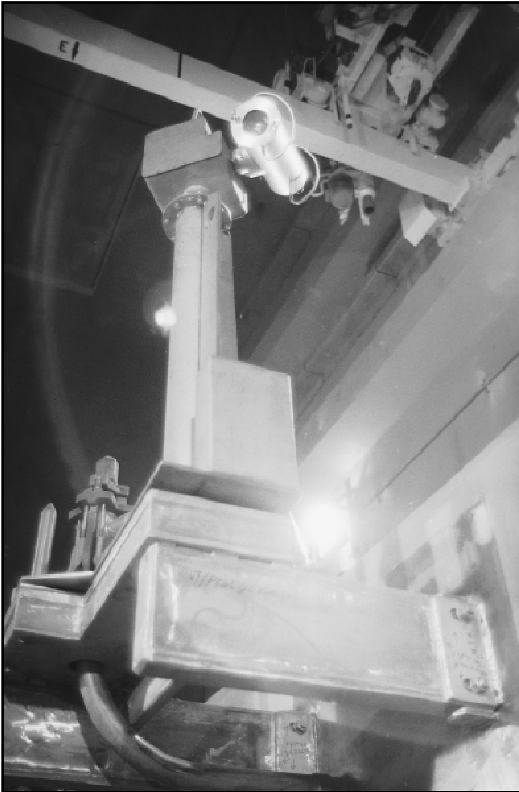
A remote monitoring camera inside the Defense Waste Processing Facility allows workers to monitor operations in the world's largest high-level nuclear waste processing facility. This facility fills canisters with high-level nuclear waste solidified in glass. The waste was generated by reprocessing operations, which extracted plutonium for use in nuclear weapons. The waste-filled canisters are stored awaiting the availability of a geologic repository for permanent disposal. Savannah River Site, South Carolina. June 15, 1993.
