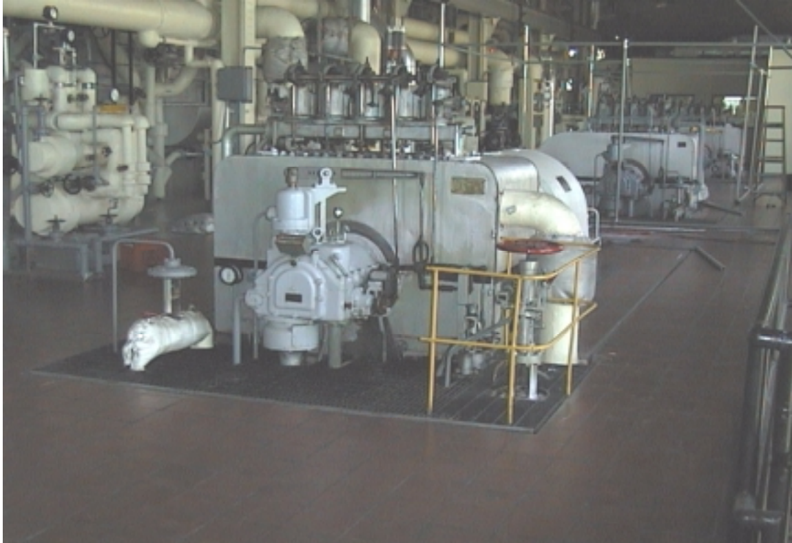
Figure 4 Parris Island Cogeneration Facility
