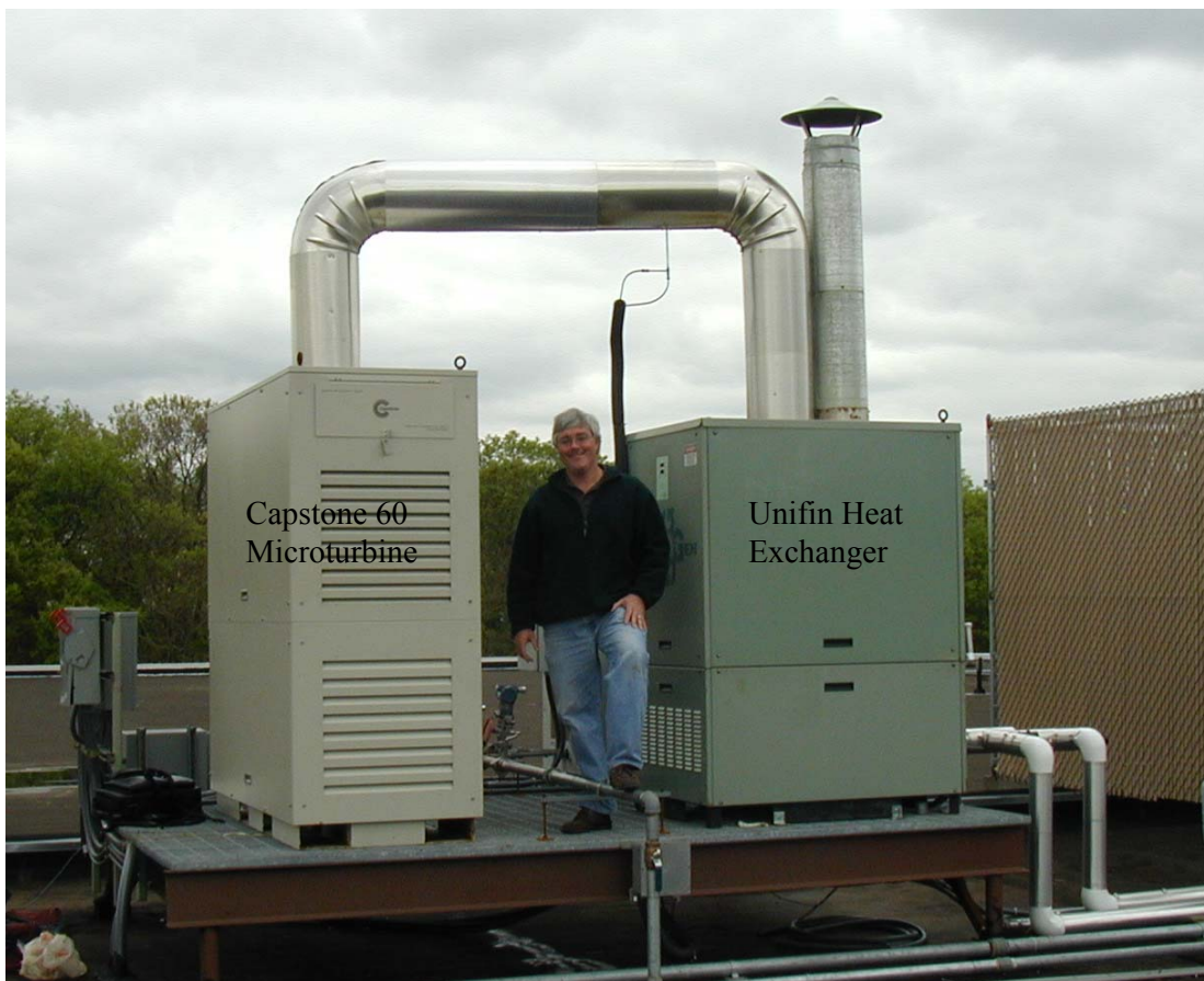
Figure 1-1. The Waldbaum's Capstone 60 Microturbine System
