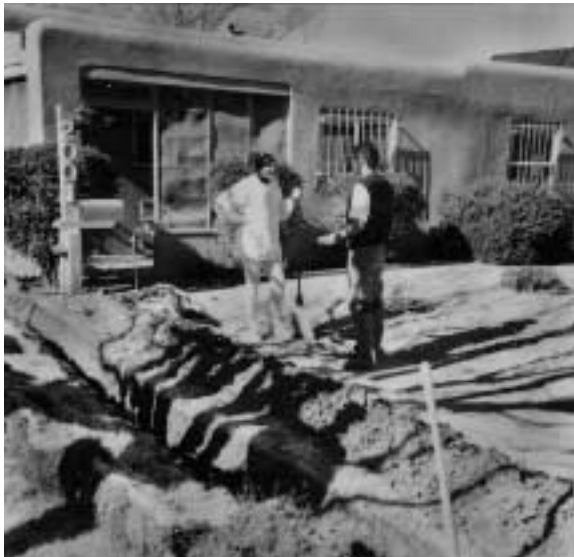
MO LOCHER and Peter Feng talk about water-leak repair at her home. Several Sandians helped install new plumbing — at no charge. Mo says she discovered what a "real family" is all about.
