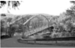
FIGURE 4 This uncommon multiple-span lenticular truss bridge carries Dutchtown Road over the Susquehanna River in Broome County and is listed in the National Register. (Courtesy of Mead & Hunt, Inc.)
