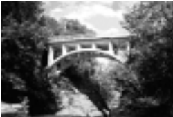
FIGURE 3 This open spandrel concrete deck arch carrying Route 30 over Mine Kill in Schoharie County was included in the field review and was determined to be eligible for the National Register. (Courtesy of Mead & Hunt, Inc.)
