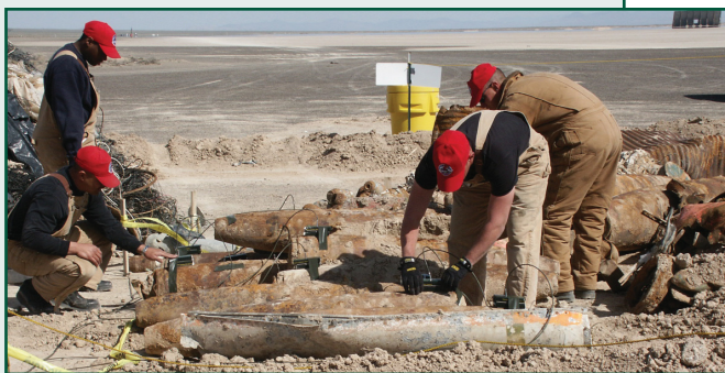
Members of the 820th Red Horse Squadron install C-4 plastic explosives during the demolition of unexploded ordnance at Antelope Lake on the Tonopah Test Range.
