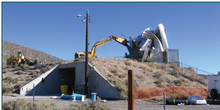
D&D activities at the Super Kukla Facility included demolition of the High Bay using hydraulic shears.
