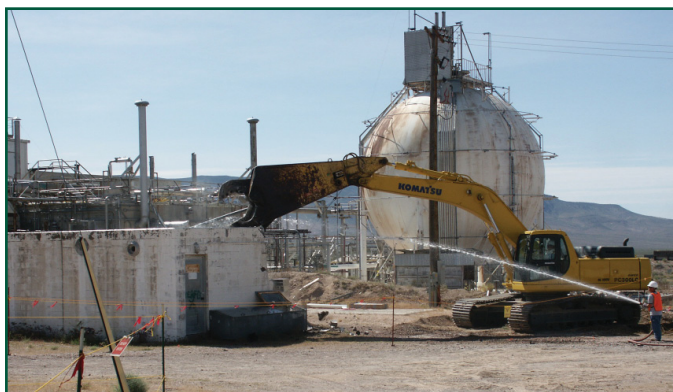
A worker sprays water for dust suppression as the hydraulic shears dismantle a building at the Test Cell A Facility on the Nevada Test Site.
