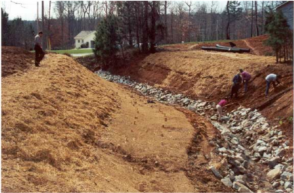
A combination of live fascines, core fabric brush mattresses live stakes, seeding and mulching has been installed.
