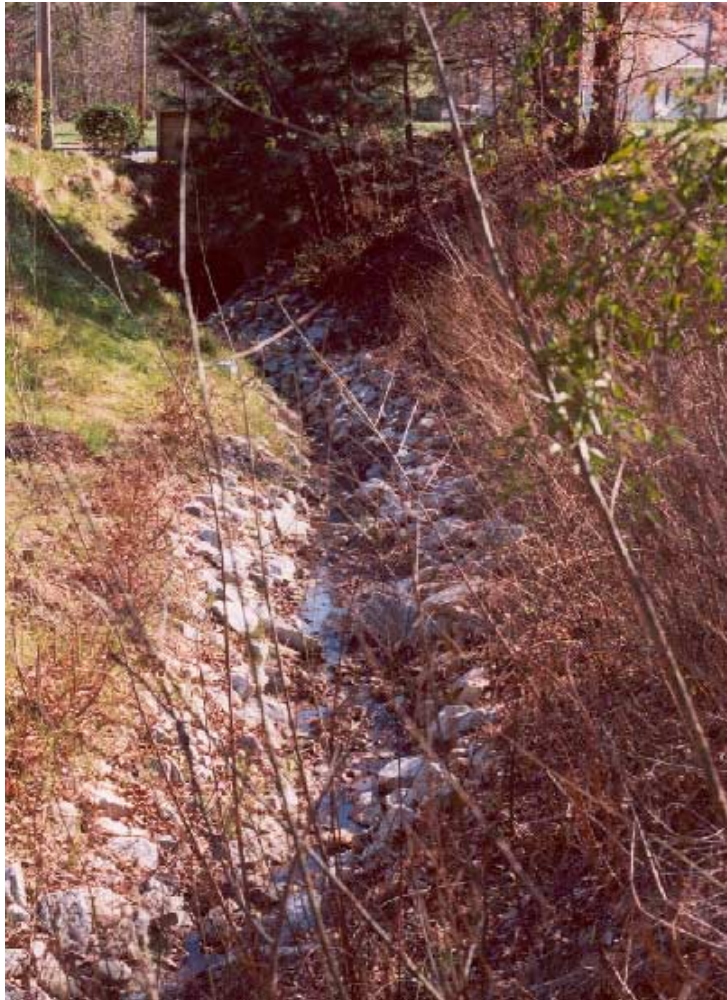
Streambank stabilization techniques shown here include tree and shrub plantings, live stakes, fascines, brush mattresses, seeding, riprap and grading and shaping.
