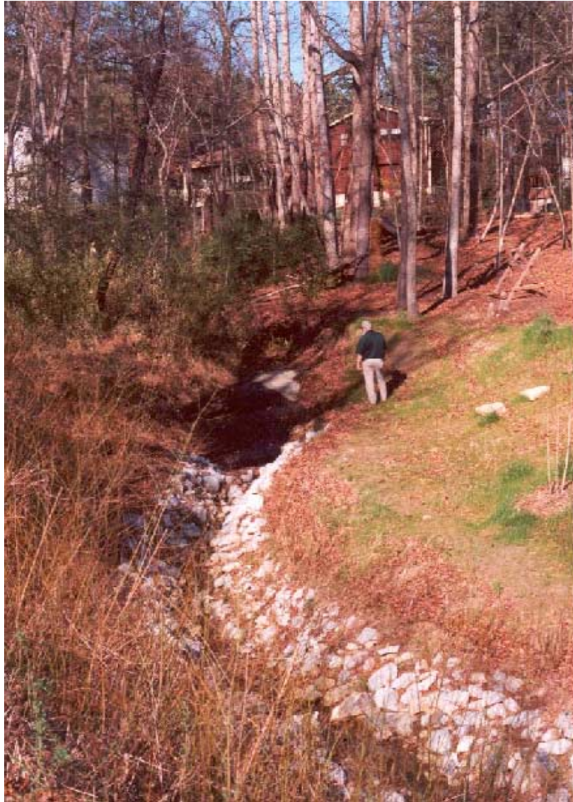
District Conservationist Steve Leslie inspects urban streambank stabilization site after one growing season.
