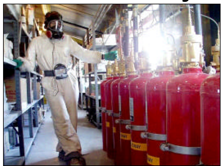
Alice Orlich eyes 16 cylinders of Foray, one of two bays of the fire-suppressing chemical that accidentally deployed in building 174 last winter.
