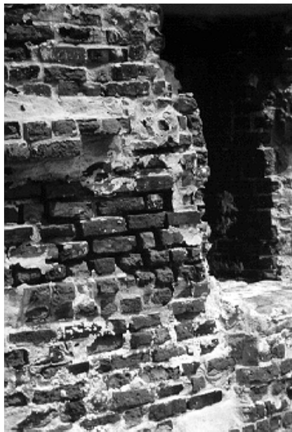
Figure 5. The coating that once protected the soft bricks of this lighthouse was not maintained; the severe deterioration required the replacement of nearly 25,000 bricks.
