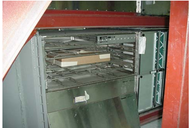
Figure G-6. 2-1200 CFM M49 Installed with HEPA Filters and Prefilters
