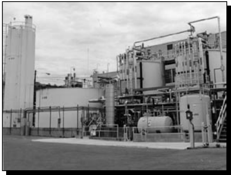
Central Neutralization Facility
