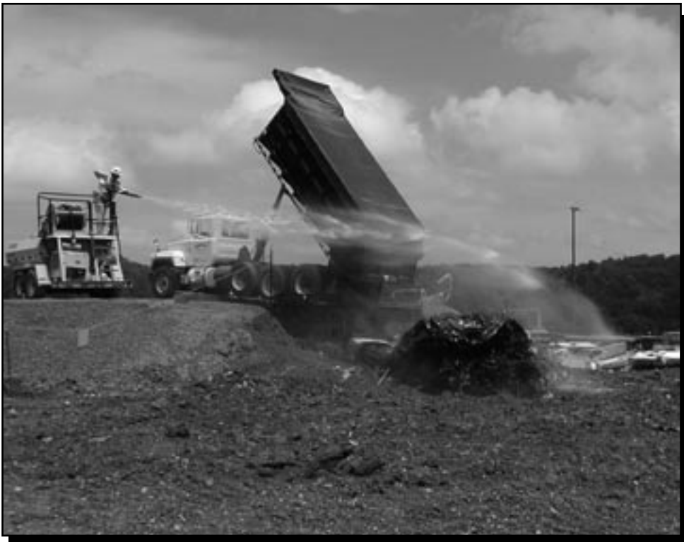
Workers spray water on a load of waste being placed in EMWWMF to suppress dust.
