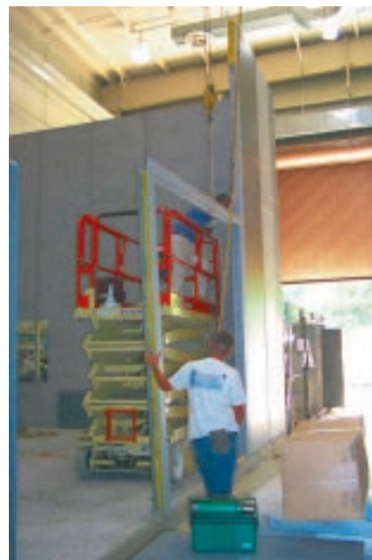
Figure 1. Access door frame being installed. The test chamber complex was assembled from prefabricated modular components.
