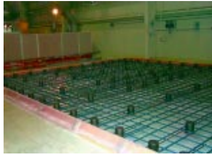
Figure 4. Test chamber seismic base with rebar and vibration isolator forms in place ready for concrete pour.
