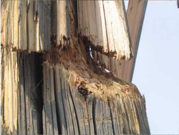
Close up of red M/R blade strike looking due west. M/R was under full power when it struck pole.
