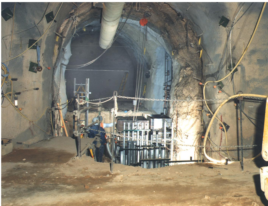
One of two experimental alcoves in the 102 minicomplex during construction. Workers are installing the utilities required to stage and diagnose subcritical tests.
