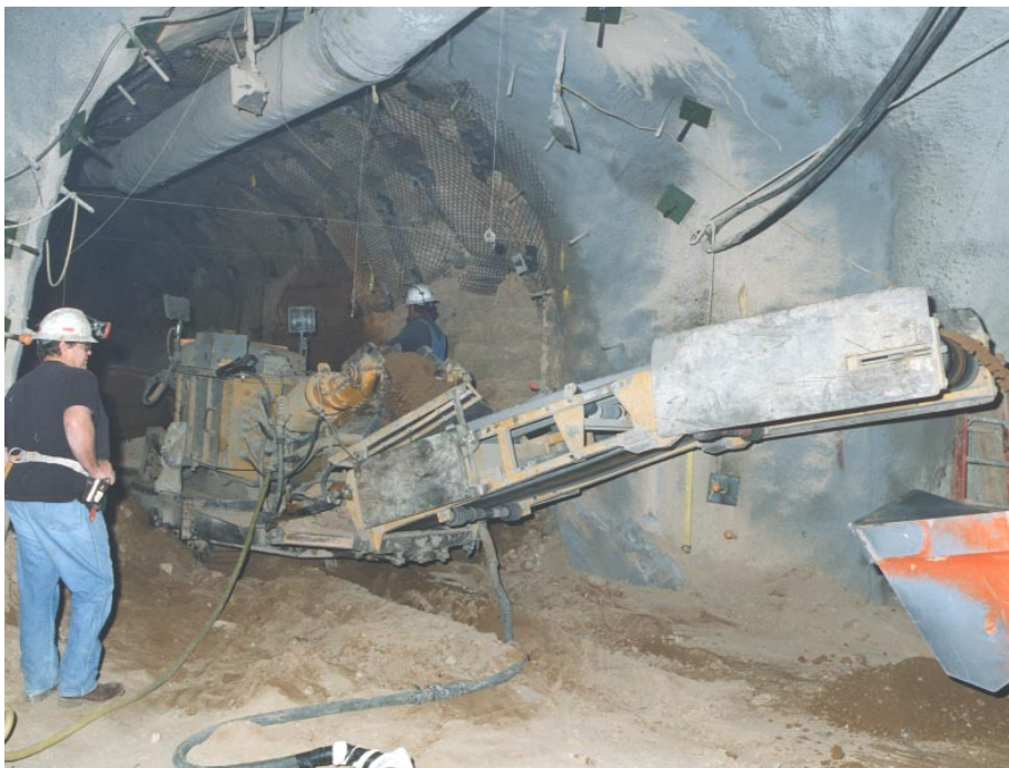
Equipment typically used for making subway tunnels was used to carve out Livermore's underground test facilities.
