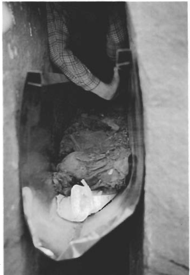
Figure 21 — View of Working Conditions within the Crevice
