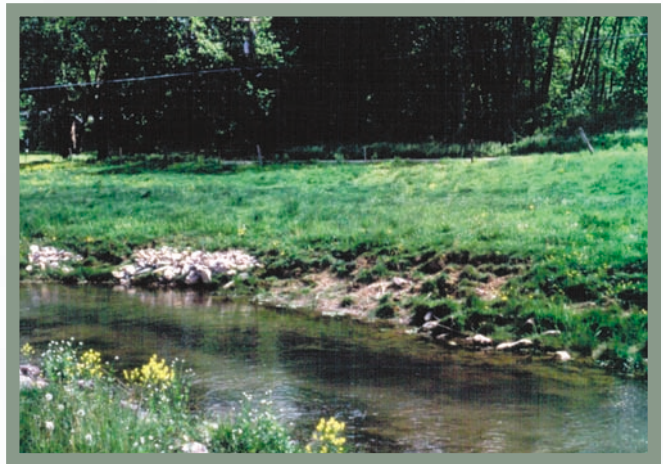
Figure 2. Some landowners put stones that they found on their fields on sections of the streambanks that were becoming eroded.
