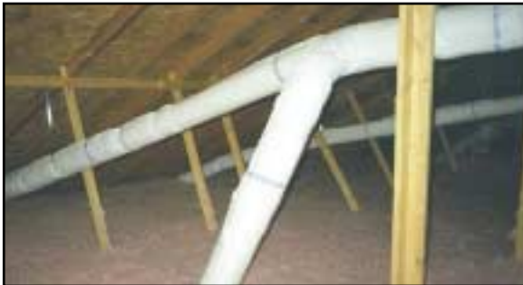
Suspended ducts are vulnerable to attic temperatures.
