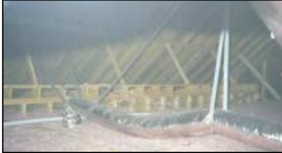
Suspended flex ducts droop between supports. The supports can restrict the air flow.
