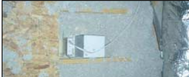
These recessed lights were IC rated but the insulation contractor was not notified.
