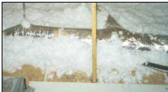
Insulation is piled up against the ducts to provide extra protection from the attic's temperatures.
