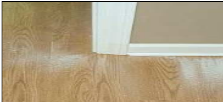
Evidence of a leaky interior wall.
