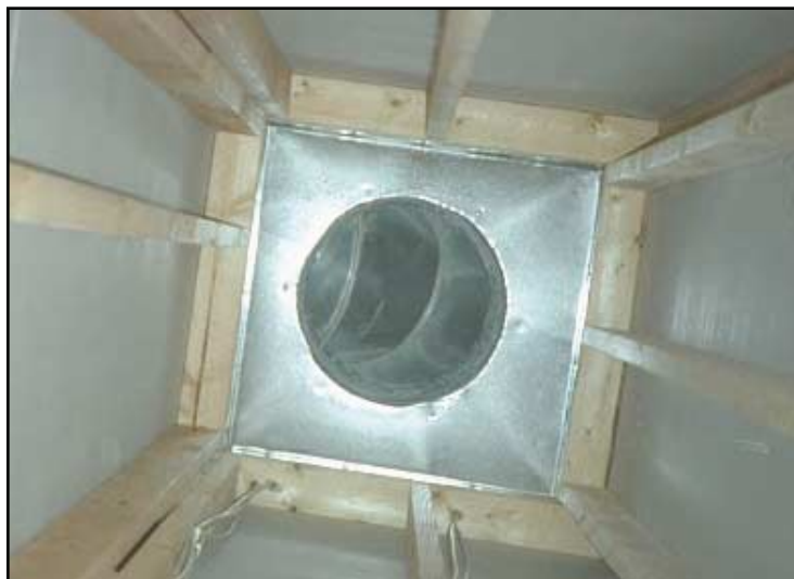
A home-made return air "duct." Note the unsealed electrical penetrations at the top that can pull down attic air into the return
