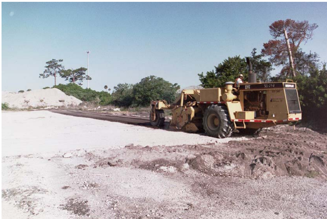
Figure 3.2 Mixing of RAP and Cemented Coquina from Phase I to form uniform subgrade for Phase II
