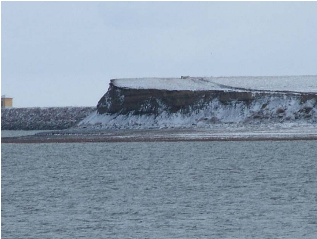
Figure 5 – Extensive eroded shoreline looking towards Belle Fourche Dam.
