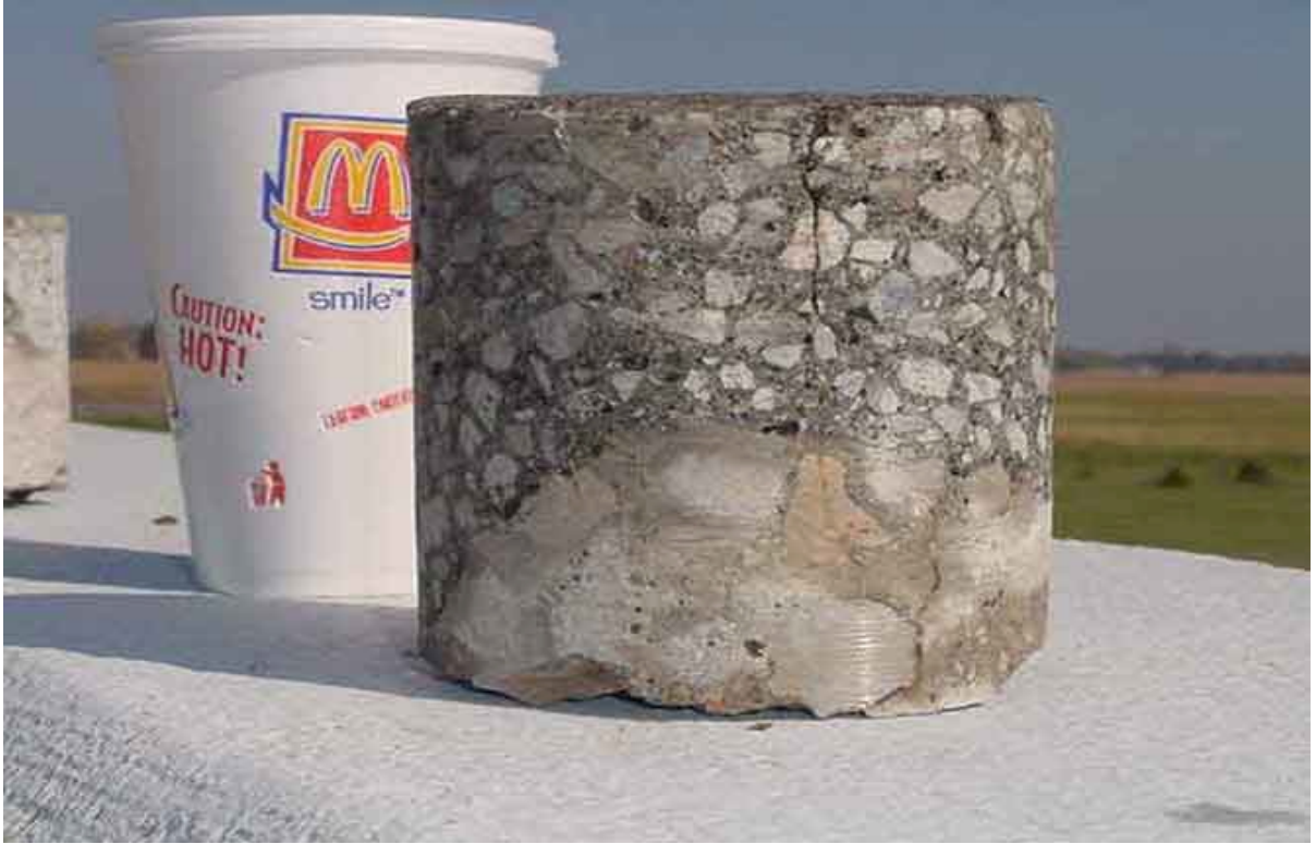
Core taken at crack
