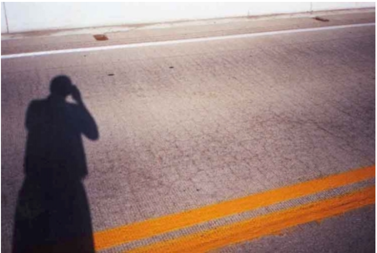
Map cracking of wearing surface
