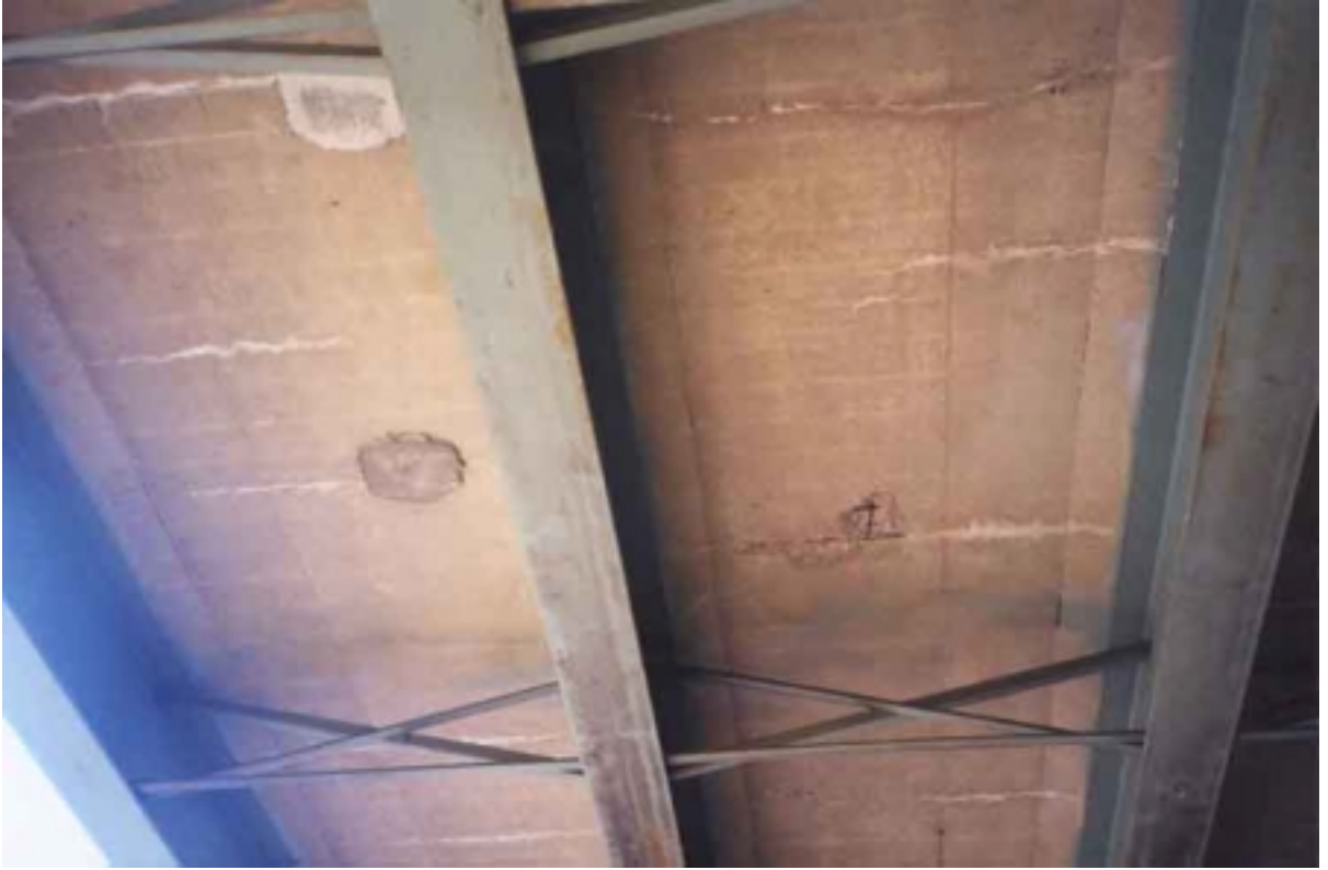
Some previous patched areas; minor spalling; transverse cracks with efflorescence
