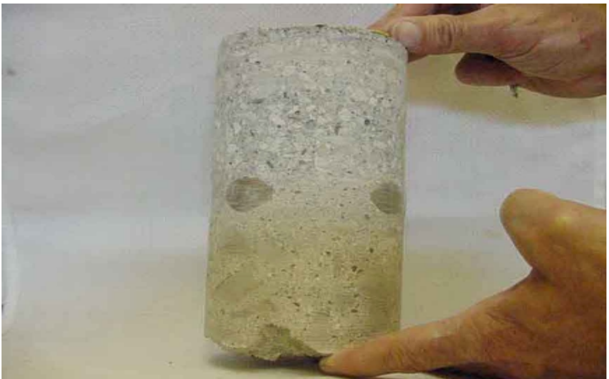
Core showing that not all reinforcing steel indicates corrosion activity
