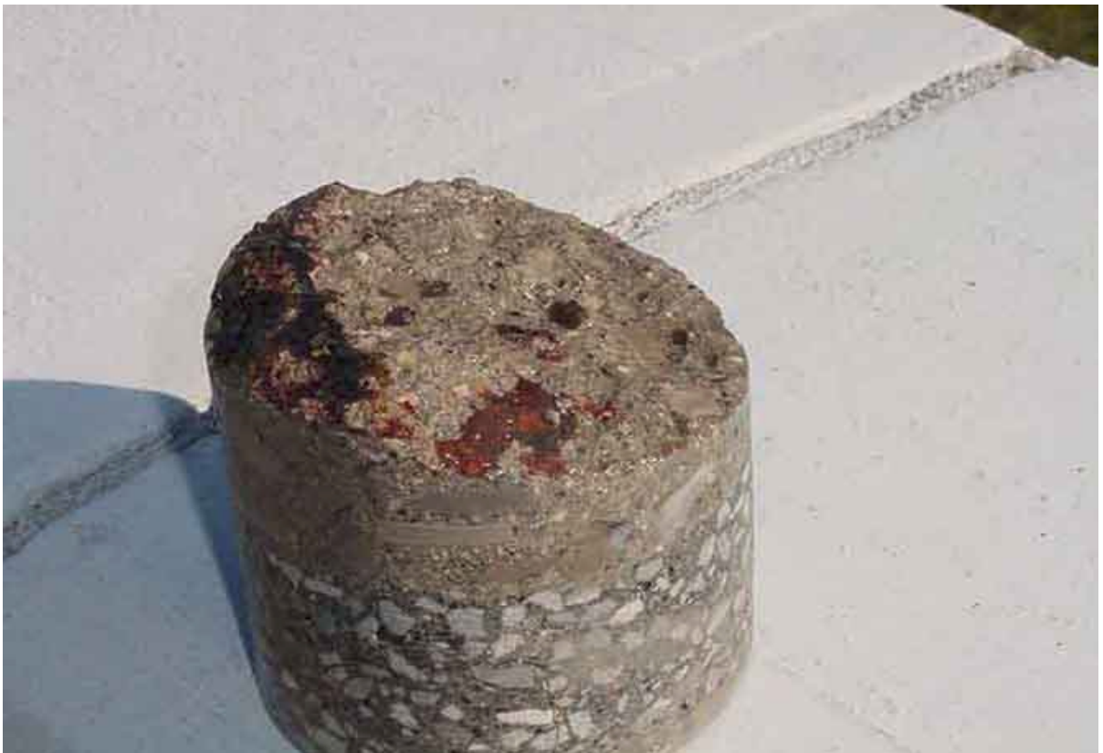
Core showing corrosion at reinforcing steel in parent concrete (upside down core)
