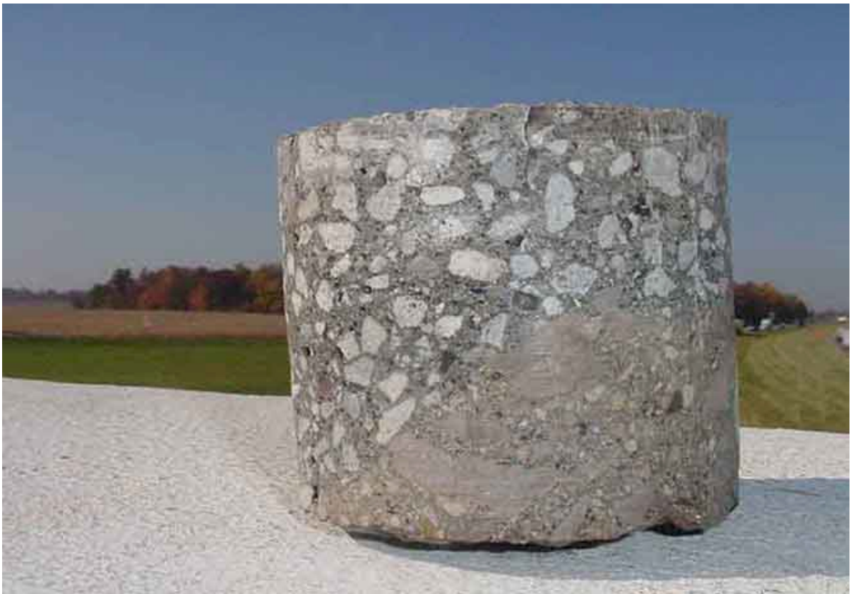
Core showing variable thickness of overlay
