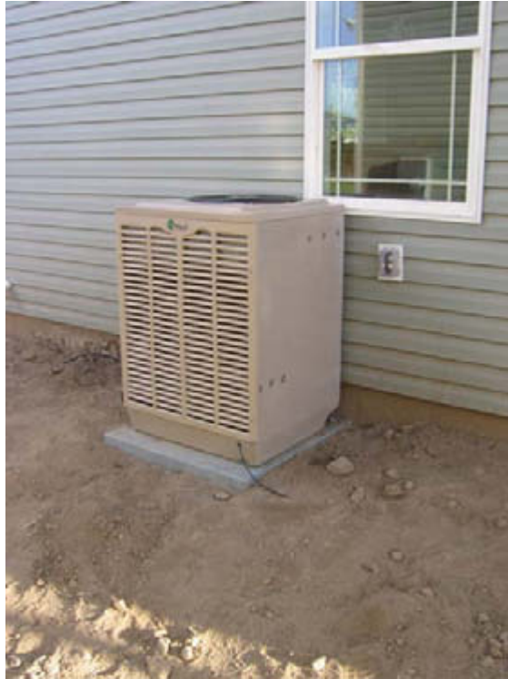
Figure 5. Freus condensing unit installed at Magna Unit 2
