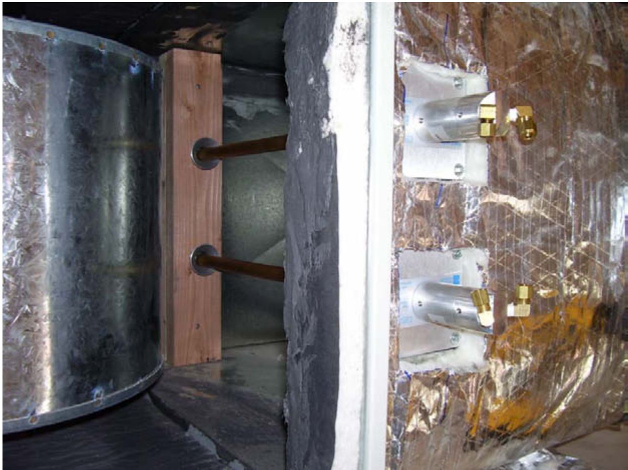
Figure 23. Pitot tube traverse airflow sensors installed at the return duct for the DiGiorgio home
