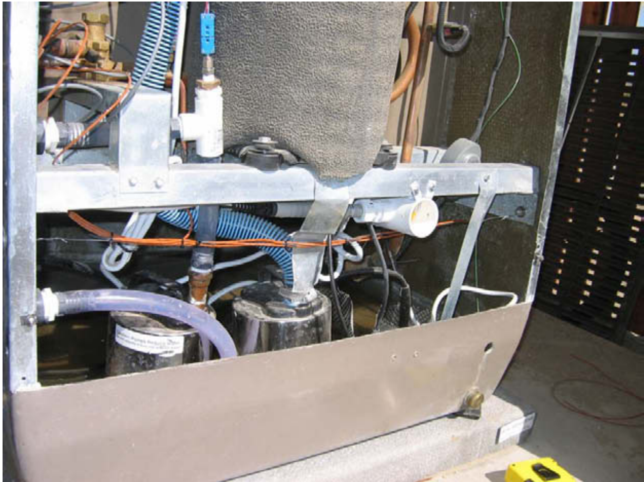
Figure 26. Thermocouple (brown wire) and Vaisala temperature and RH sensors (white PVC shield + gray sensor) installed at Freus air intake, grill removed
