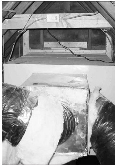
The photo shows an attic installation of a Phoenix evaporative cooler by Direct Drive Service. The cooler is installed close to the fresh-air intake and moves air into 24-inch-diameter supply ducts. The ducts are well insulated (improving energy performance and reducing noise) and relatively short, as they typically feed conditioned air into an upstairs hallway. Intake air ducts range from 28 x 42 inches down to 24 x 36 inches; the smaller size will accommodate a 3,000 CFM evaporative cooler. The cooler is suspended from trusses and uses vibration isolators at top and bottom. In the interests of safety, an electric cutoff is installed close to the unit, so that it can be maintained without risk of shock.
