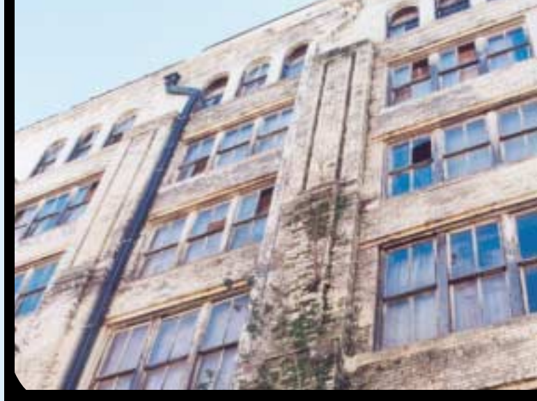
The historic Awalt Building was in serious disrepair when Slingshot Communications purchased the building for adaptive reuse.
