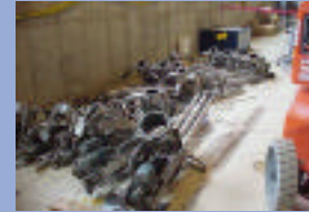
Manipulator arms, tools that had been used in the past to handle irradiated items, were removed from the walls of the Hot Cells.
