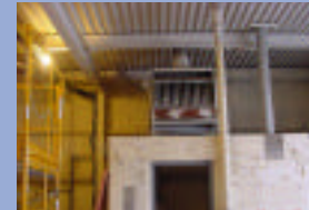
A varnish was applied to the surface of this air vent and other fixed equipment to prevent dust-like loose contamination from becoming airborne during removal.
