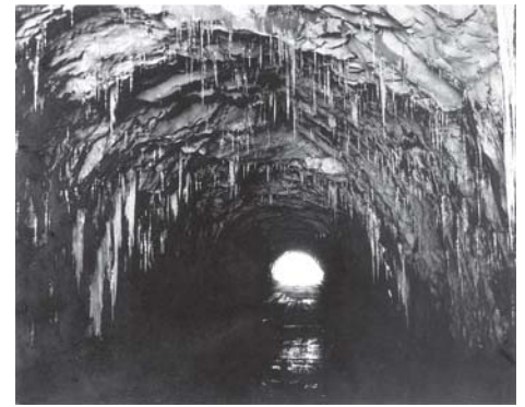
Interior of Marys Rock Tunnel: This early interior view of the tunnel indicates the winter conditions before the concrete lining was installed in 1958-1959. Today, the north portal still exhibits icicles that, on occasion, can reach ten feet in length.
