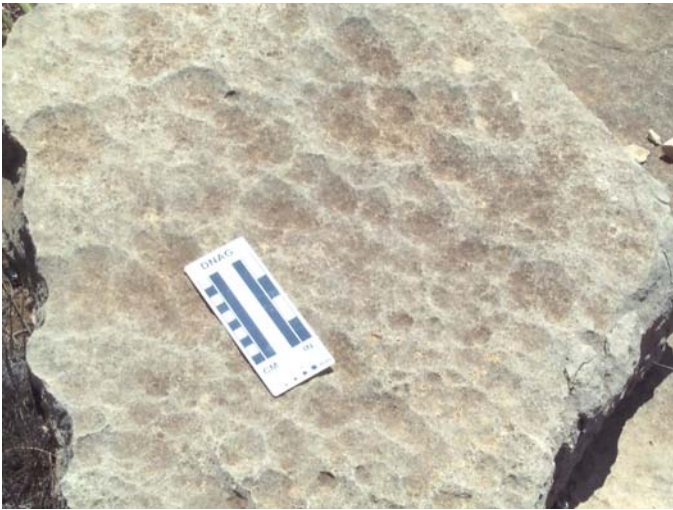
Some areas exhibit larger, more rounded pitting.
