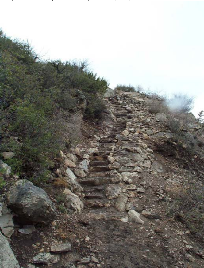
AFTER PHOTO: A series of built-in steps and other measures were employed to correct the problems. (NPS Photo by Diane Dobos-Bubno)
