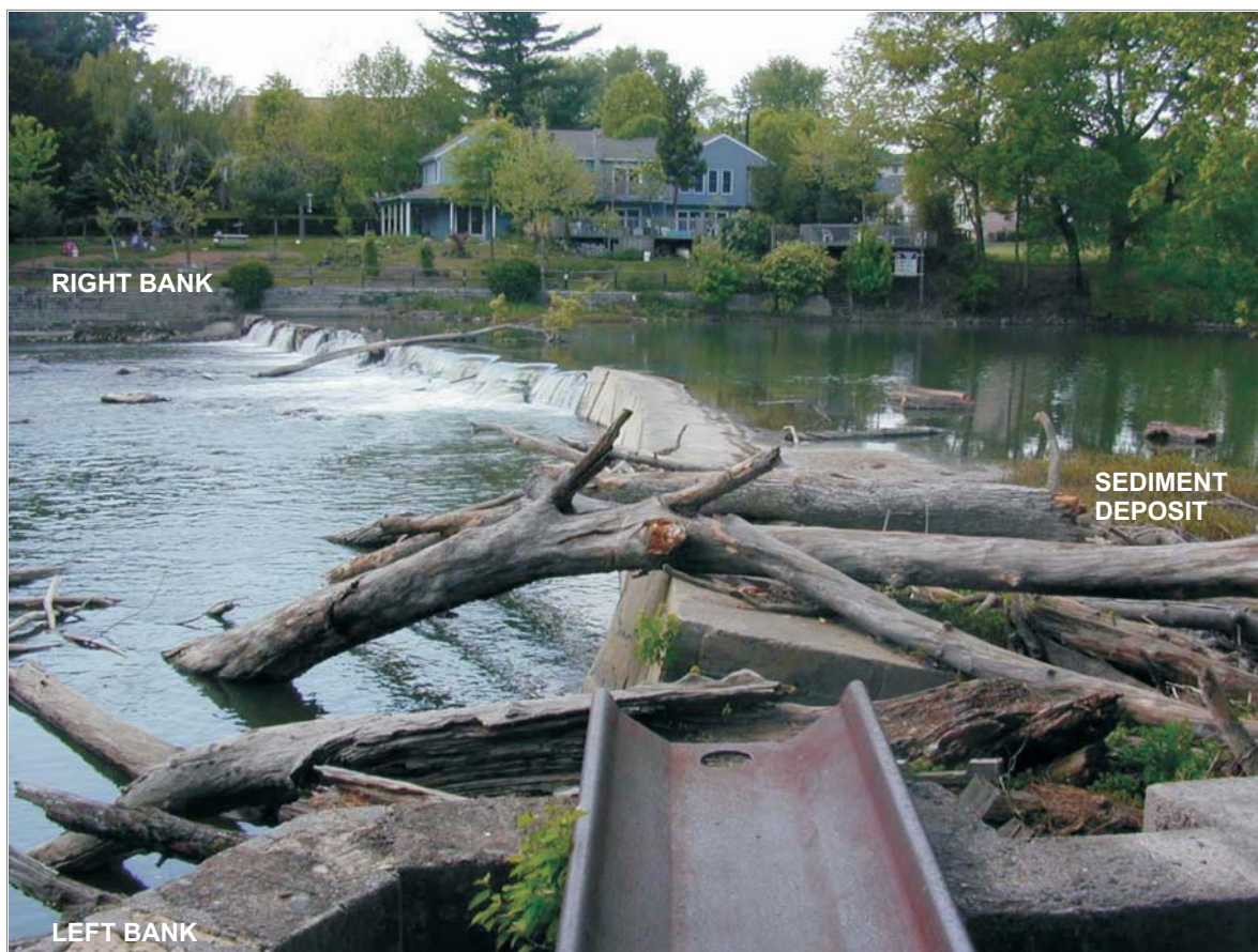
Figure 2. Conodoguinet Creek flowing over Good Hope Mill Dam, a 6-foot high, 220-foot wide concrete structure constructed on bedrock over 100 years ago to power a former mill, Cumberland County, Pennsylvania. (Photographed by J. Kent Crawford, U.S. Geological Survey, on May 21, 2001).
